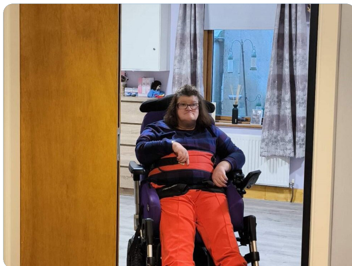
Purchased installation of automated doors, providing independent access between the bedroom, ensuite, and the rest of the home.
